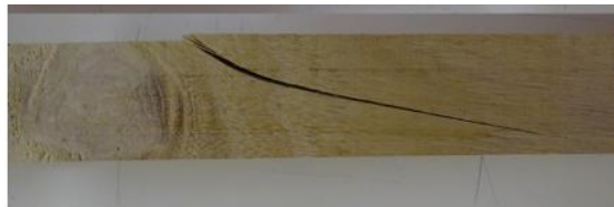
Figure 34 Wood knot where cracks form systematically
